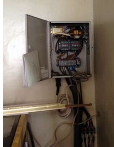
Figure: Electric board connecting the generator with the electrical installation (here: ICU generator room, 1 st general hospital)
